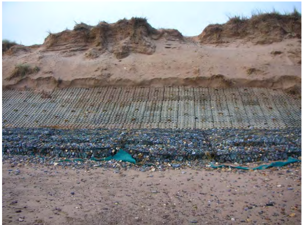
Figure 6-26: Erosion of the Dawlish dunes observed after the severe storm event on 9/10/2010.
