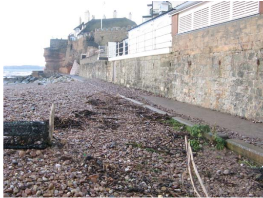
Figure B6: Debris and shingle on walkway
