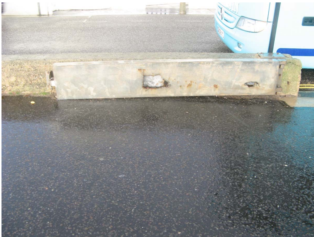
Figure 3-10 A low level concrete wall with intermittent flood barriers is located along the landward edge of the promenade at Sidmouth
