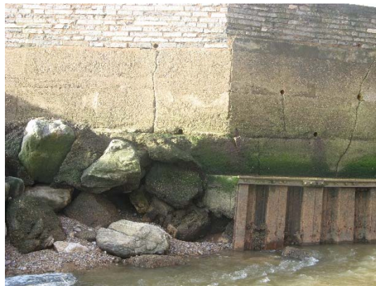
Figure F13: Sheet pile wall mass concrete scour
