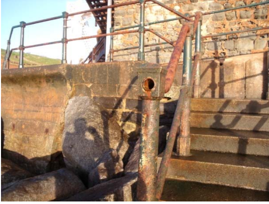
Figure A7: Corroded hand railing
