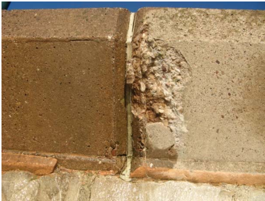
Figure D3: Spalling at expansion joints
