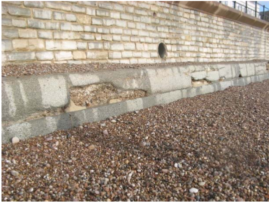
Figure E1: Badly damaged apron
