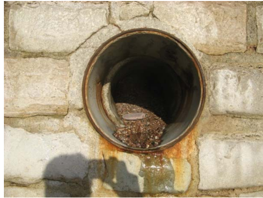
Figure D2: Blocked outfall
