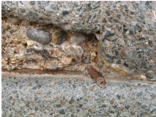
Figure E3: Exposed protruding reinforcement
