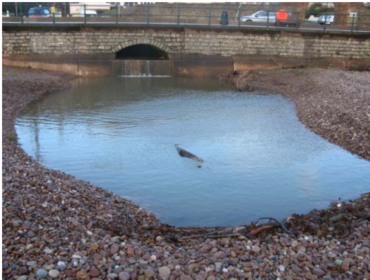
Figure C3: Large outfall and water ponding
