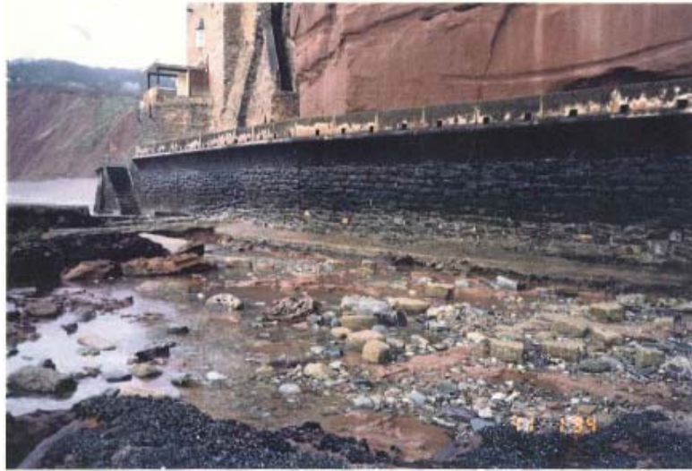
Figure 2-8 1957 seawall and the encountered erosion during the 1994 January inspection (from Posford Duvivier, 1994)
