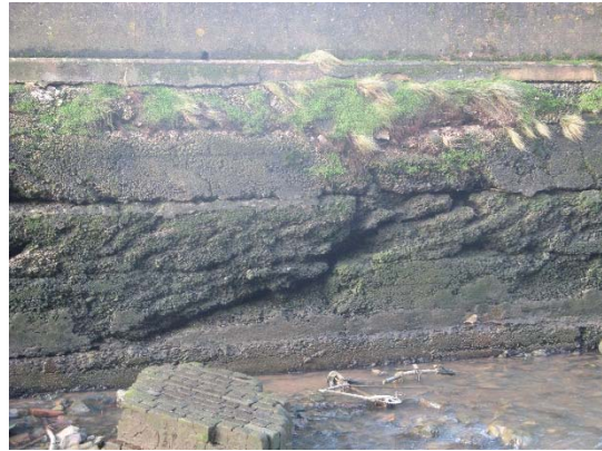
Figure G6: River wall spalling/erosion
