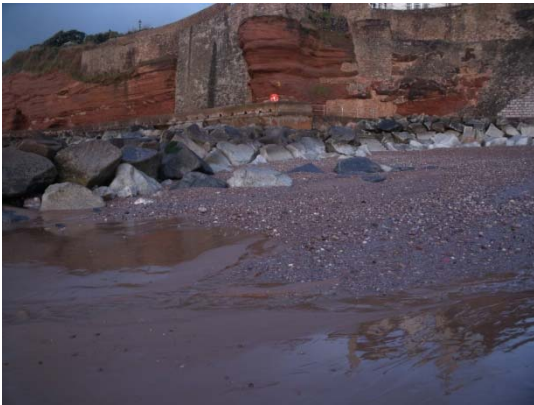
Figure A17: East groyne flank, displaced rocks
