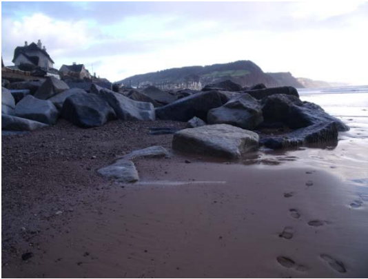
Figure A15: West groyne flank, displaced rocks
