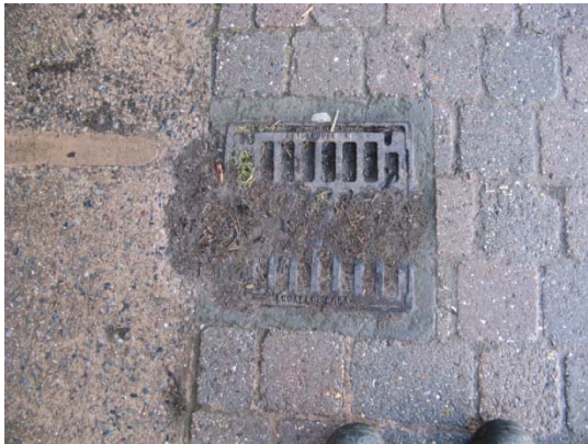
Figure B7: Blocked gully
