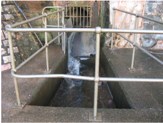
Figure B5: Outfall and screen
