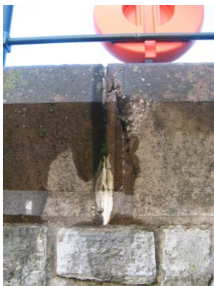
Figure C5: Cracking and missing sealant on coping
