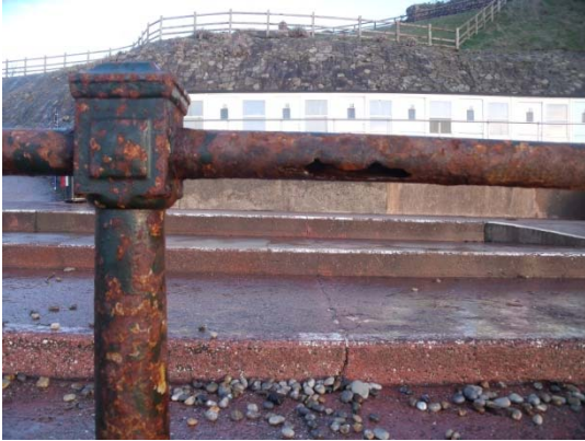
Figure A1: Corrosion holes in hand railing
