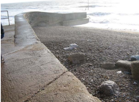
Figure F9: West groyne flank, no hand railing
