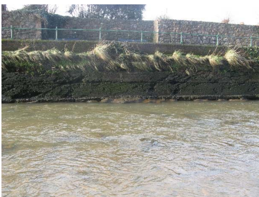
Figure G9: River wall undermining
