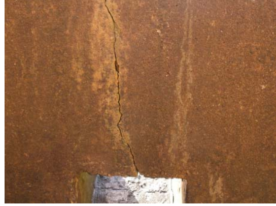
Figure A8: Cracking at drainage outlet
