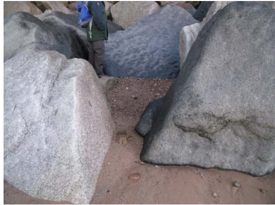
Figure A14: Large voids between rock armour
