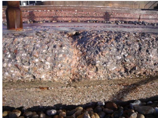
Figure A4: Damaged seawall coping
