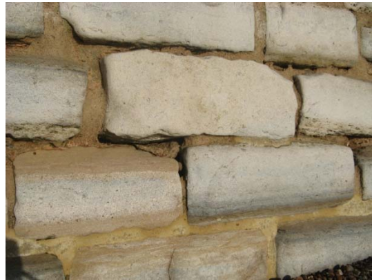
Figure D4: Masonry joints filled with mortar
