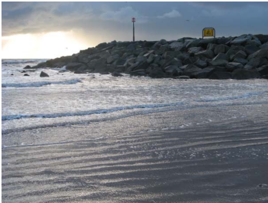
Figure B17: Displaced rocks on western breakwater
