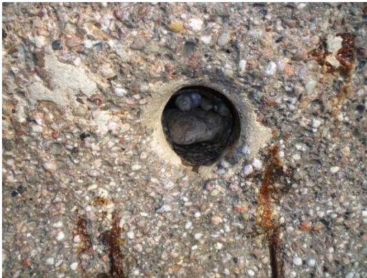
Figure A3: Blocked outfall
