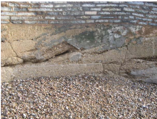
Figure F7: Holes and cracking
