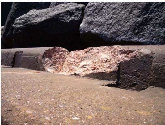
Figure A9: Coping damage
