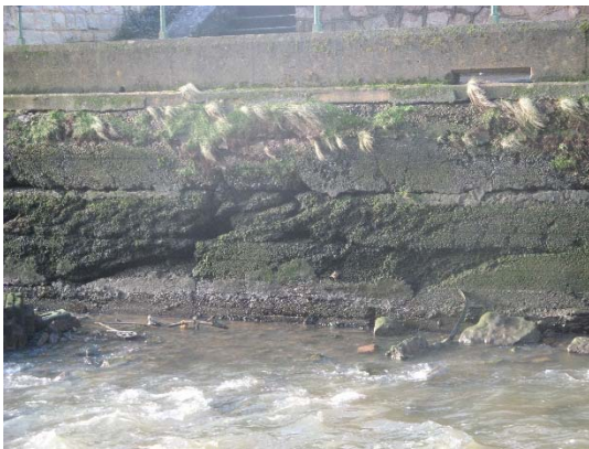
Figure G7: River wall spalling/erosion
