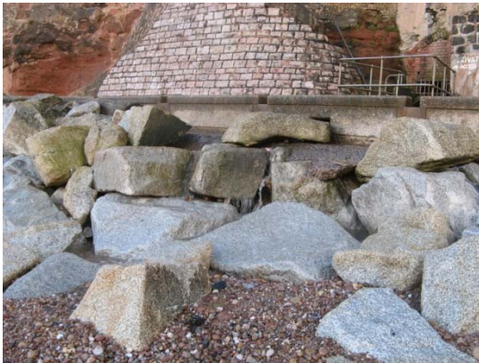
Figure B13: Displaced rocks and shingle infill at toe
