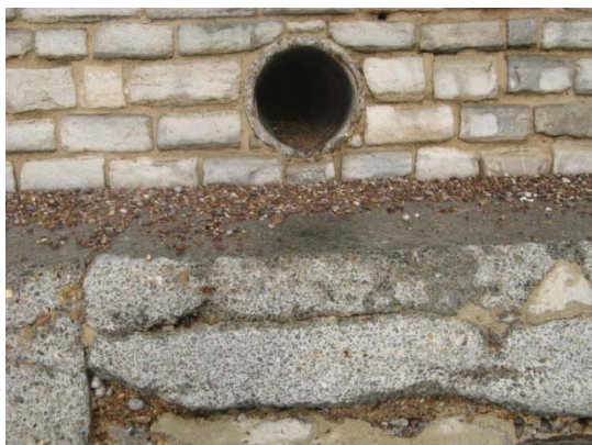
Figure E5: Blocked outfall
