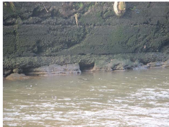
Figure G8: River wall undermining
