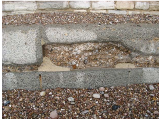
Figure E2: Badly damaged apron
