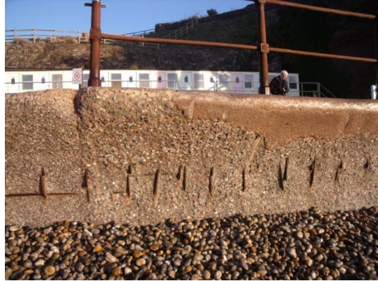
Figure A2: Exposed reinforcement and abrasion
