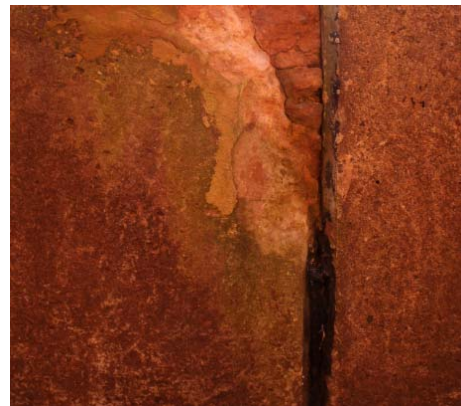
Figure A10: Spalling at expansion joints
