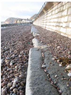
Figure D5: Cracking and abrasion to apron
