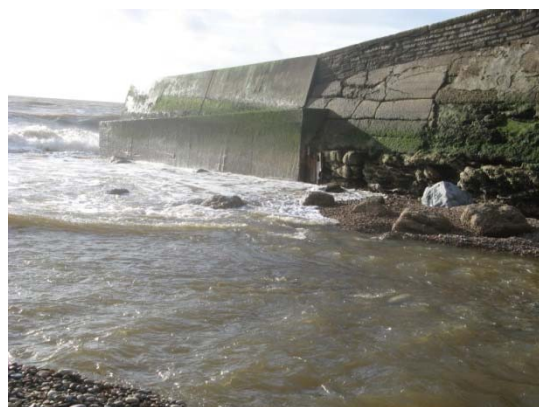
Figure F10: East groyne flank
