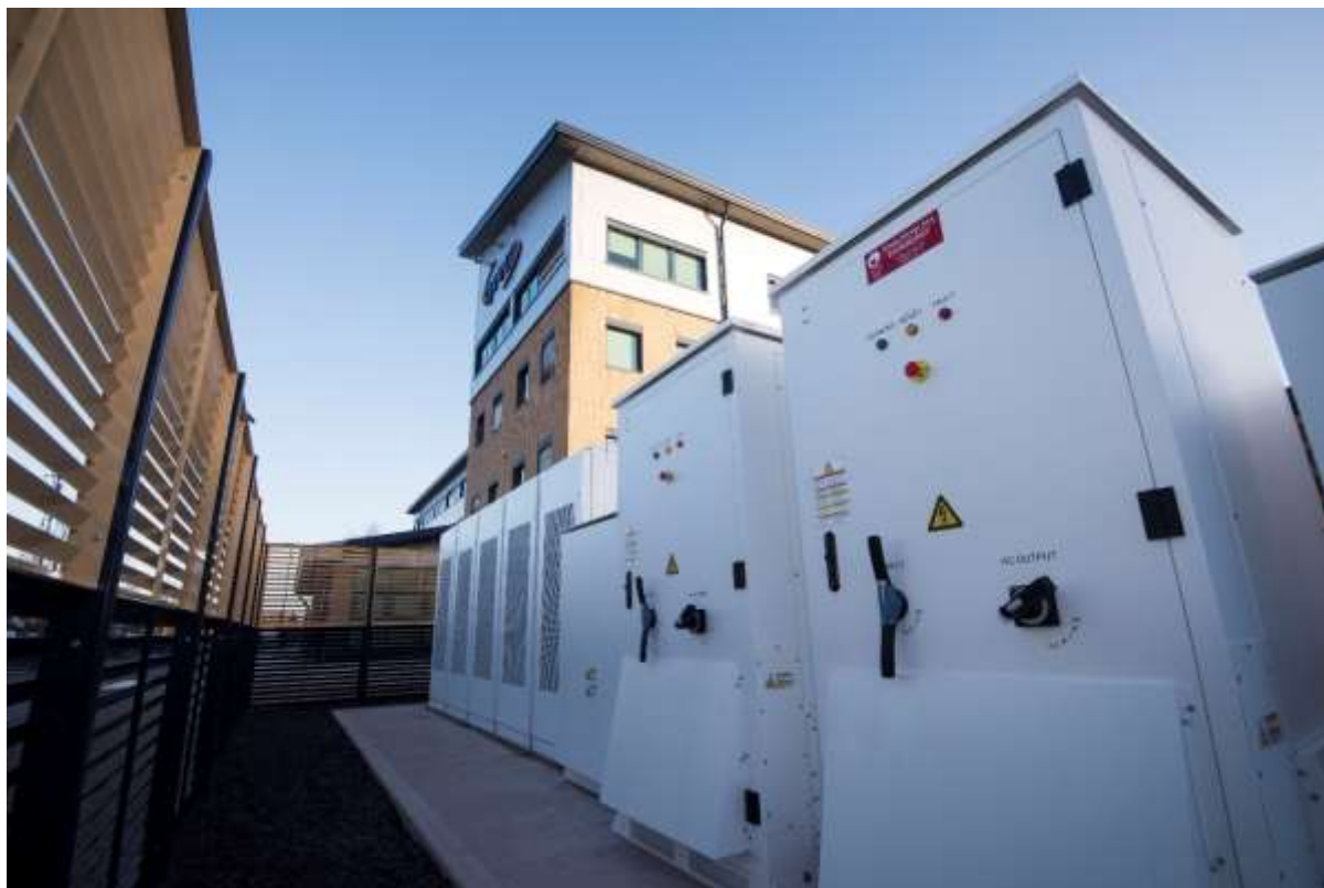
FIGURE 9. Example battery storage facility
