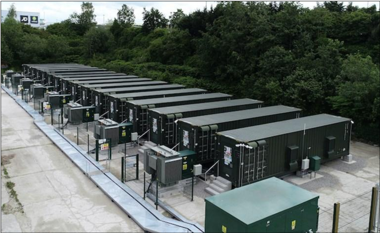
FIGURE 9 Example Anesco battery storage facility (Source: Anesco)
