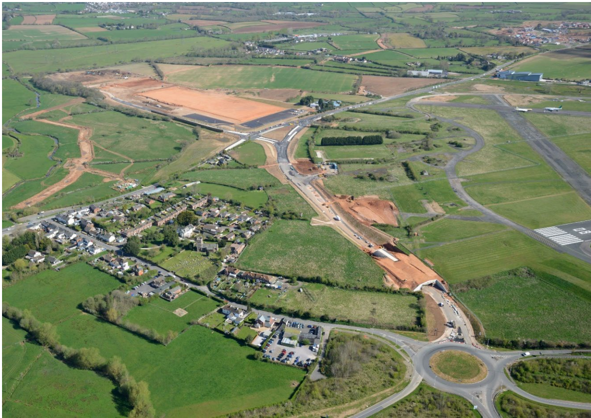
Figure 44: Clyst Honiton Bypass and Lidl Site under construction with Clyst Honiton Village in the foreground.
