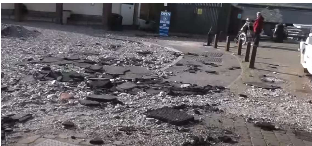
Figure 2: Example of historic damage to promenade road area.
