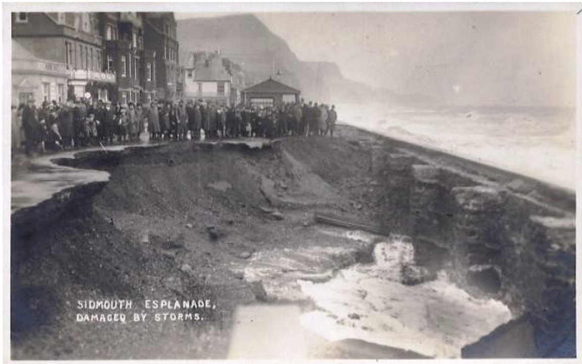
Figure 18, when large holes developed behind the seawall during 1920s storms, causing extensive flooding and damage to the road and services.
