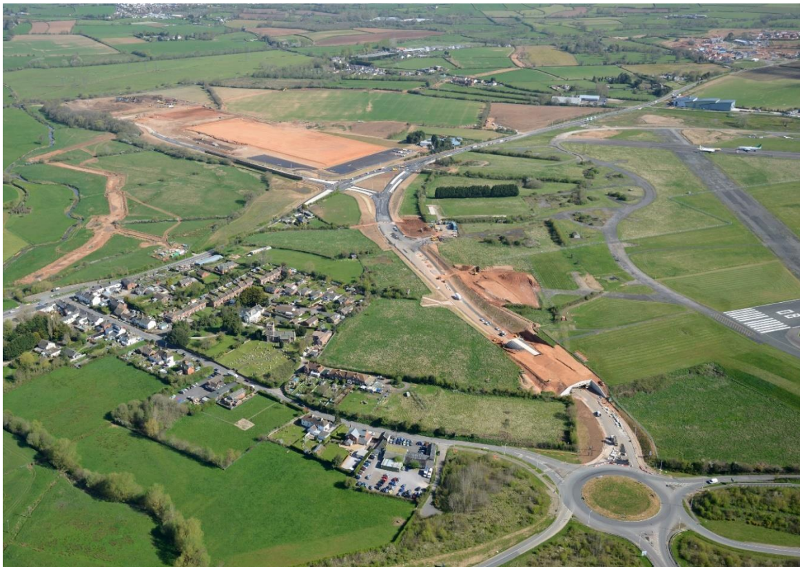
Figure 48: Clyst Honiton Bypass and Lidl Site under construction with Clyst Honiton Village in the foreground.
